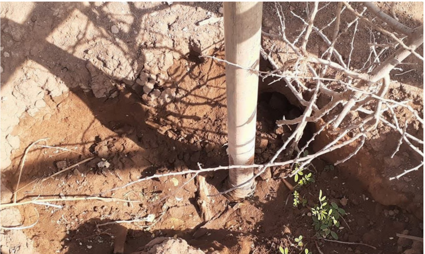
Lanqood borehole, Wajir, mainline piping system needs repair - partially-functional © Adaptation Consortium
