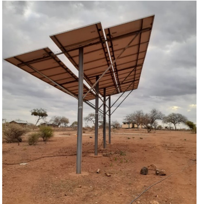
Yatta borehole, Wajir, solar panel technical problem - partially-functional © Adaptation Consortium
